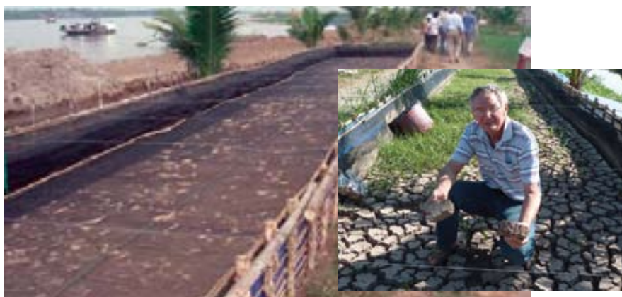
Sludge pens remove solids from dredge discharges before their release to the effluent canal.
