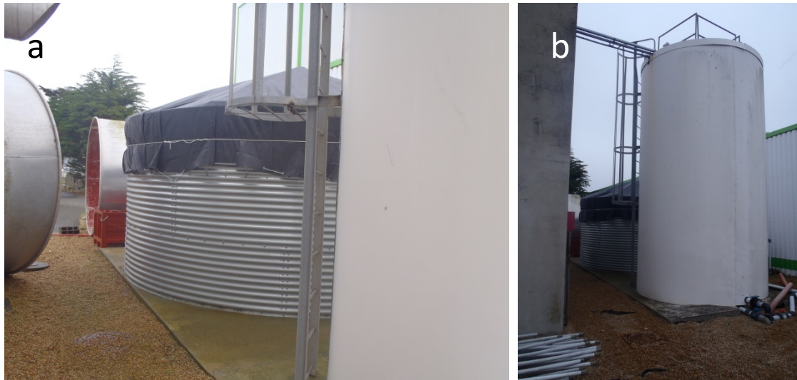
Figure 2.2 a) and b) Tanks for storage of seawater at CEVA. Total capacity of 45 m 3 (a) and 20 m 3 (b).
