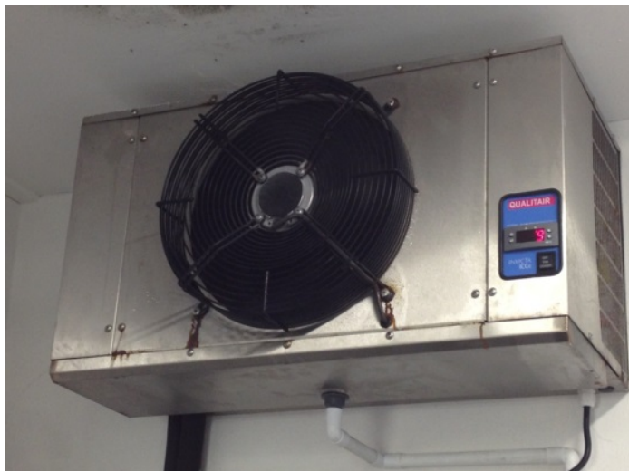
Figure 2.4. Qualitair Invicta ICCe Refrigeration unit attached to external wall of hatchery in QUB.
